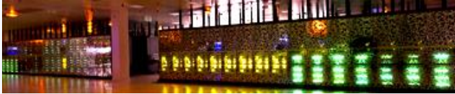
CEA data centre supporting digital services
