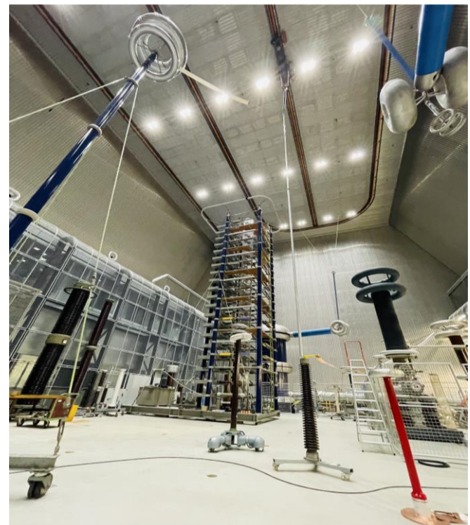
Tuning the 4000 kV DCVD of TU Delft with the VSL LI measuring system
