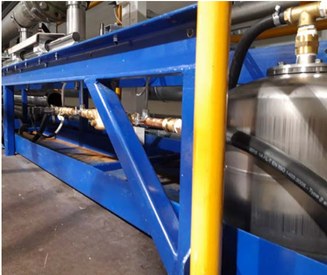
Inlet and pressure vessel
