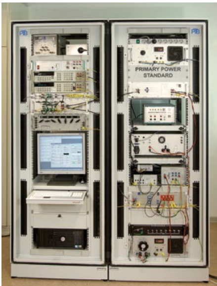
PTB's primary standard for electrical power.
