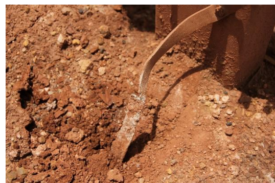
Figure 1: Ground electrode affected by salt corrosion
