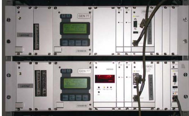
Figure 3. New NTP servers ptbtime1 (lower) and ptbtime2 (upper).
