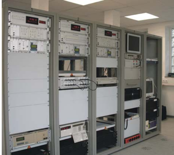
Figure 1. New electronic control during construction. As a detail, one can see in racks 1 to 3 the three signal generators and temporarily only two atomic frequency standards.
