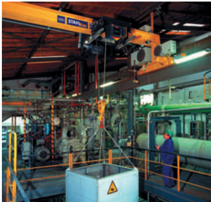
Figure 1: Explosion protected crane installation
