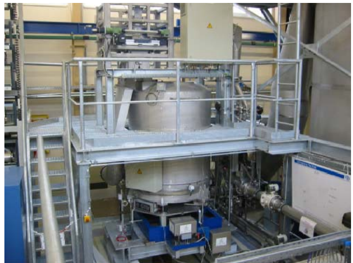
b) 3-tons weighing system of the calibration plant ( above )
