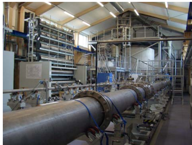
Fig. 2 View of the calibration hall (calibration lines with the weighing system in the background)
