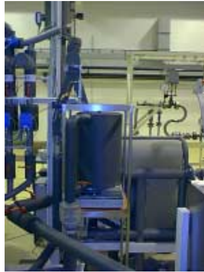
Picture 7: Weighing system 4
